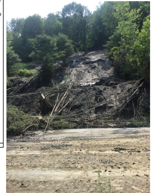
Landslide on VT-62, Barre, VT
